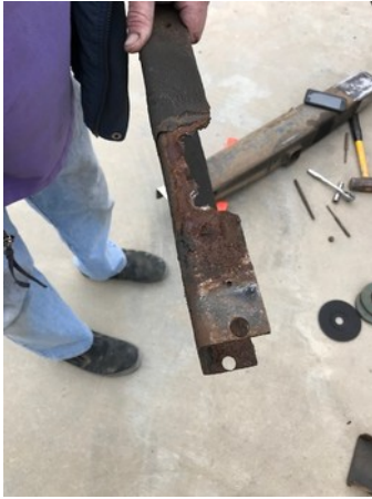
Here is a photo of one side of the hitch receiver mount where the hitch receiver cross member was supposed to be welded to it. It had ripped away.
